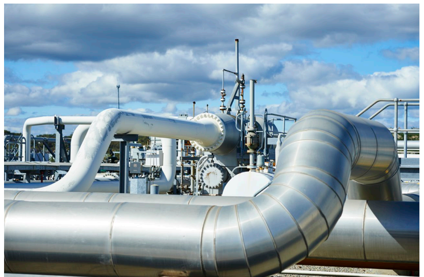
Figure 9.11: Compressor Station 10 in Kwinana
