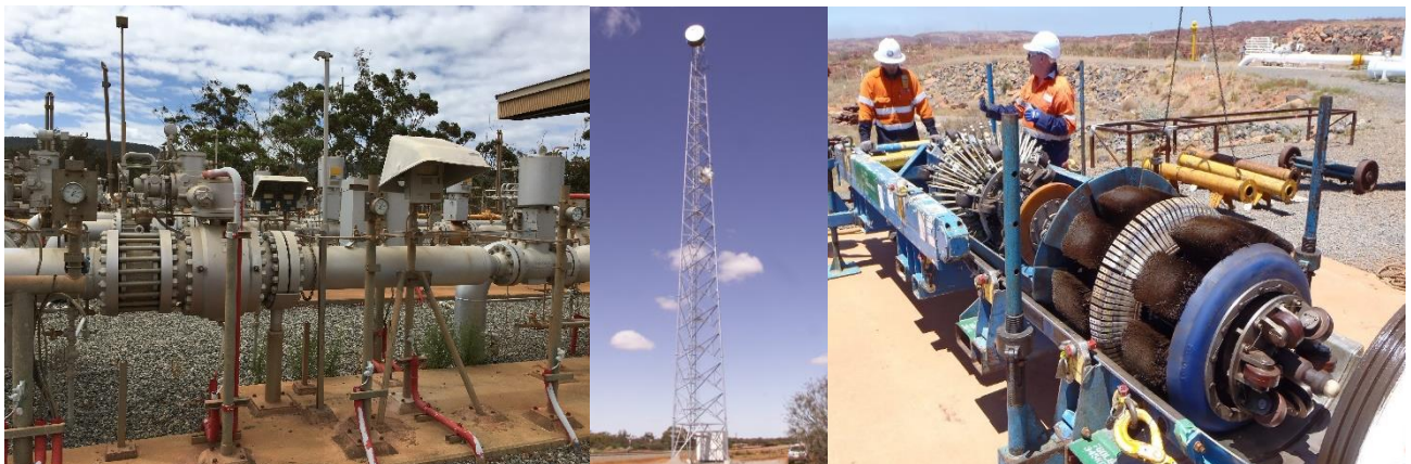
Figure 8.12: Alcoa Wagerup meter station, a telecommunications tower and pigging of the pipeline in 2018
